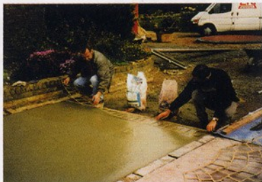
Step 1 Lay concrete in normal way and apply first line of Stencil.
